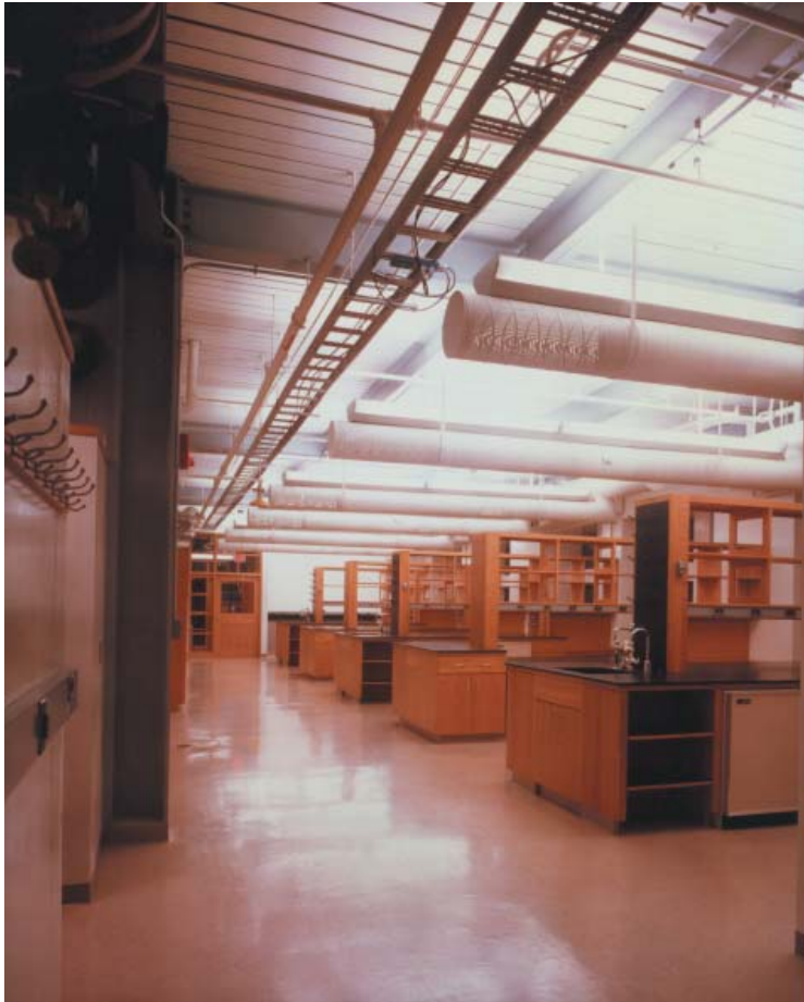
Typical open lab space in the Lewis Thomas Laboratory for Molecular Biology at Princeton University. The ceiling equipment was left exposed to expedite access to and maintenance of pipes, ducts, and cables.
